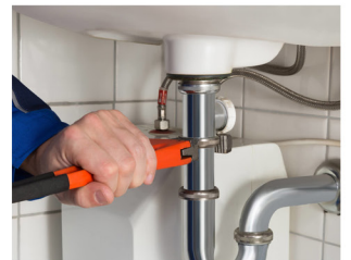
Plumbing: U.P.V.C. plumbing pipes
